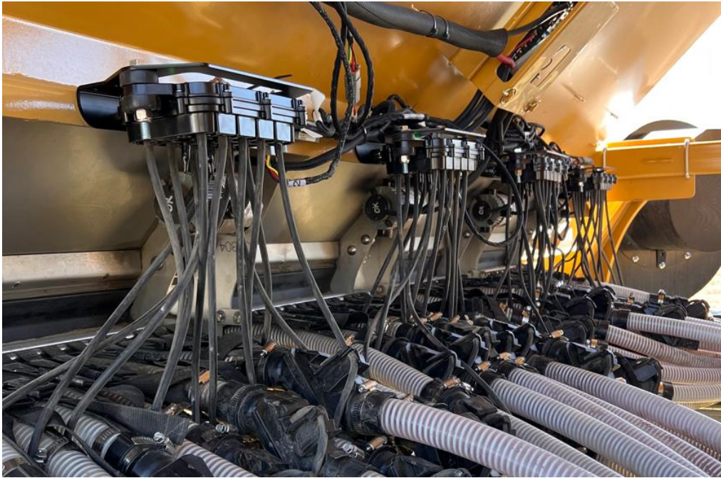
Figure 14: ECU installed on an SR-750
